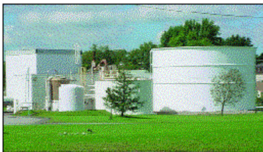
An onsite water treatment plant is part FMC's extensive groundwater remediation program.
